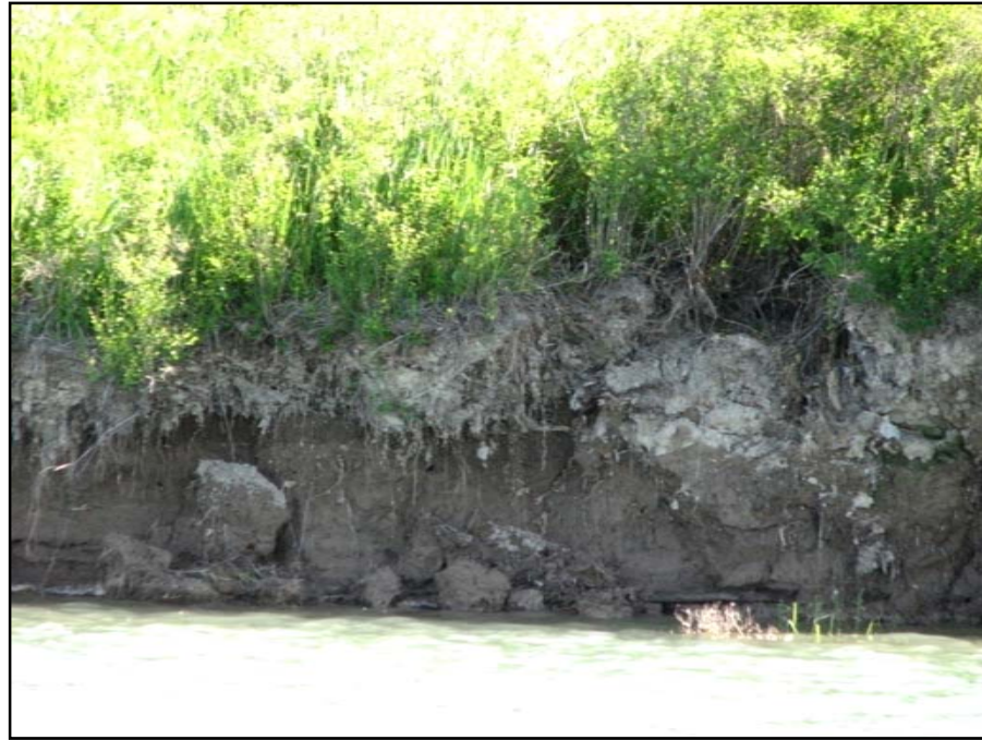
Figure 19. Saturated bank failure, Flathead River.
