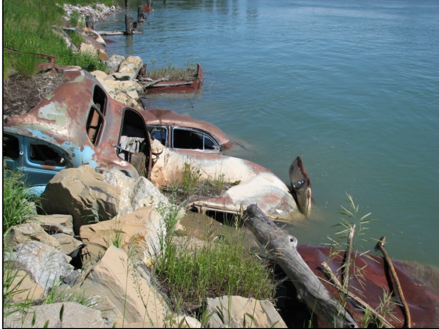
Figure 49. Typical car revetment, Flathead River; note pilings in background from failed COE wood plank revetment.
