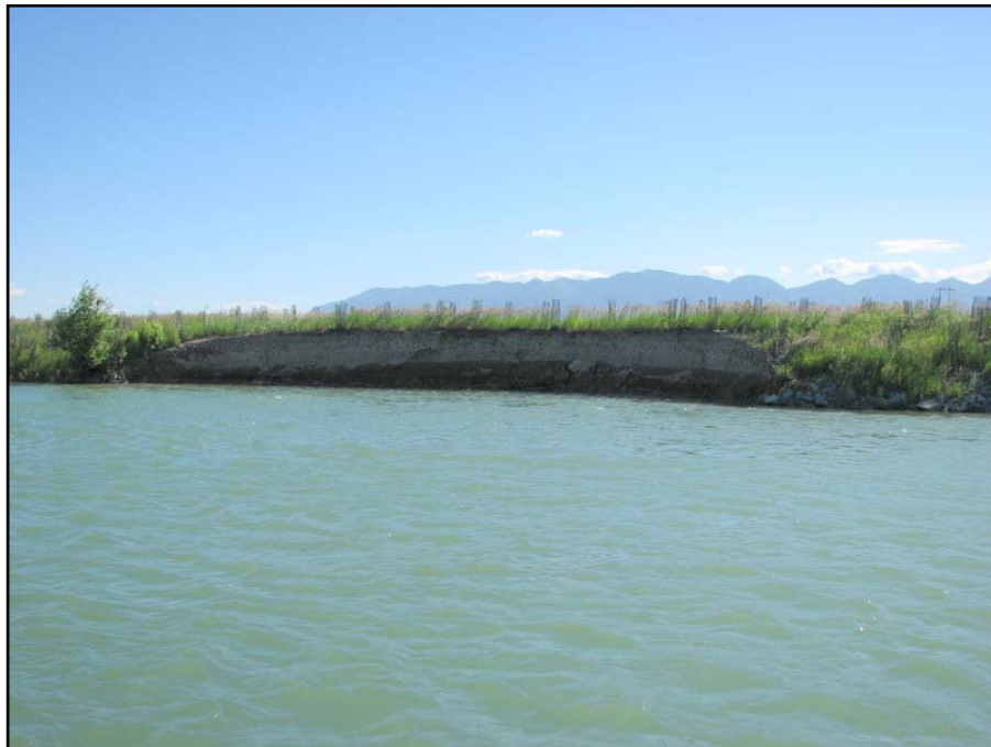
Figure 16. Severe scallop erosion of previously-armored bank, Flathead River.
