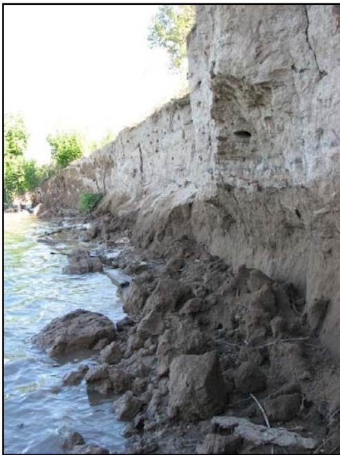
Figure 18. Lower bank undercutting, Flathead River.
