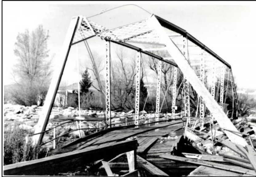
Figure 8. Bridge damage caused by 1963 Ice jam on Gallatin River near Logan (billingsgazette.com).
