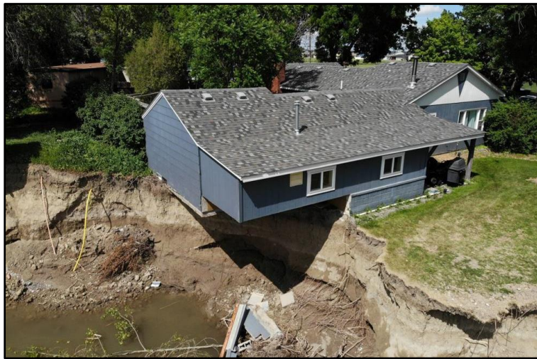
Figure 5. Billings Montana home located on ground mapped out of the Yellowstone River floodplain that was undermined in June of 2019 (Billings Gazette).
