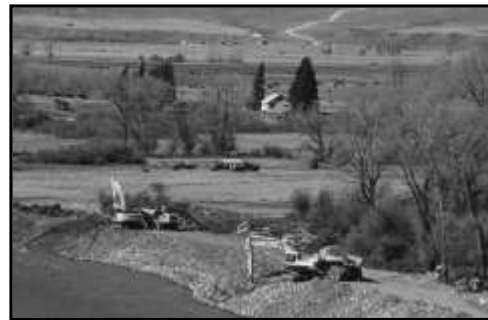
Photo 47. Post flood activity. Photo by J. Bailey.
