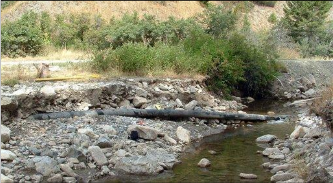
Figure 3. Exposed section of ConocoPhillips gasoline pipeline on Beaver Creek near York, Montana showing exposure from both lateral movement and vertical downcutting. ( http://ravallirepublic.com )
