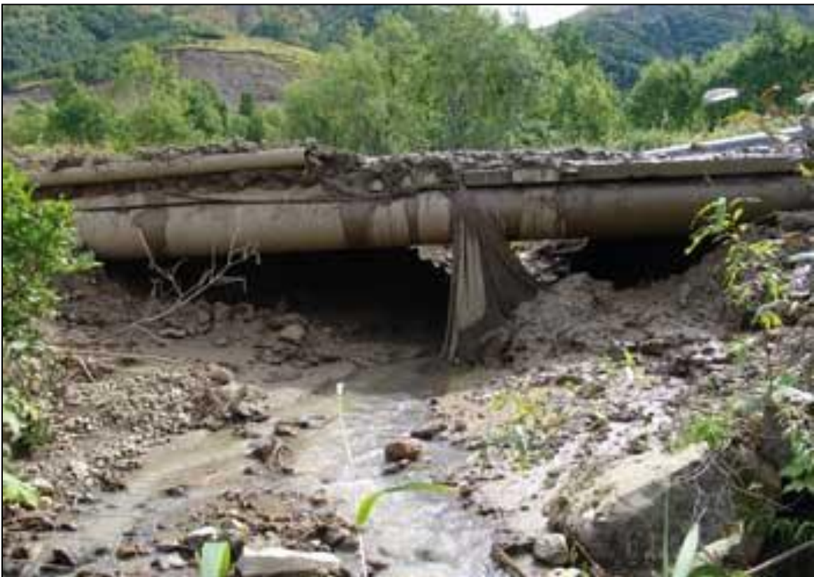
Figure 4. Pipeline exposed from vertical bed degradation, Travyanaya River, Russia. ( http://www.sakhalin.evinronment.ru )
