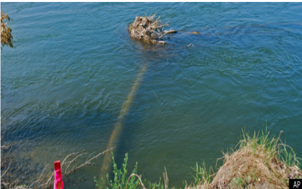
Exposed pipeline at risk of being ruptured.
