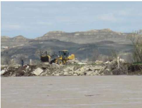
Removing concrete rubble off the river bank before it sloughs into the river.
