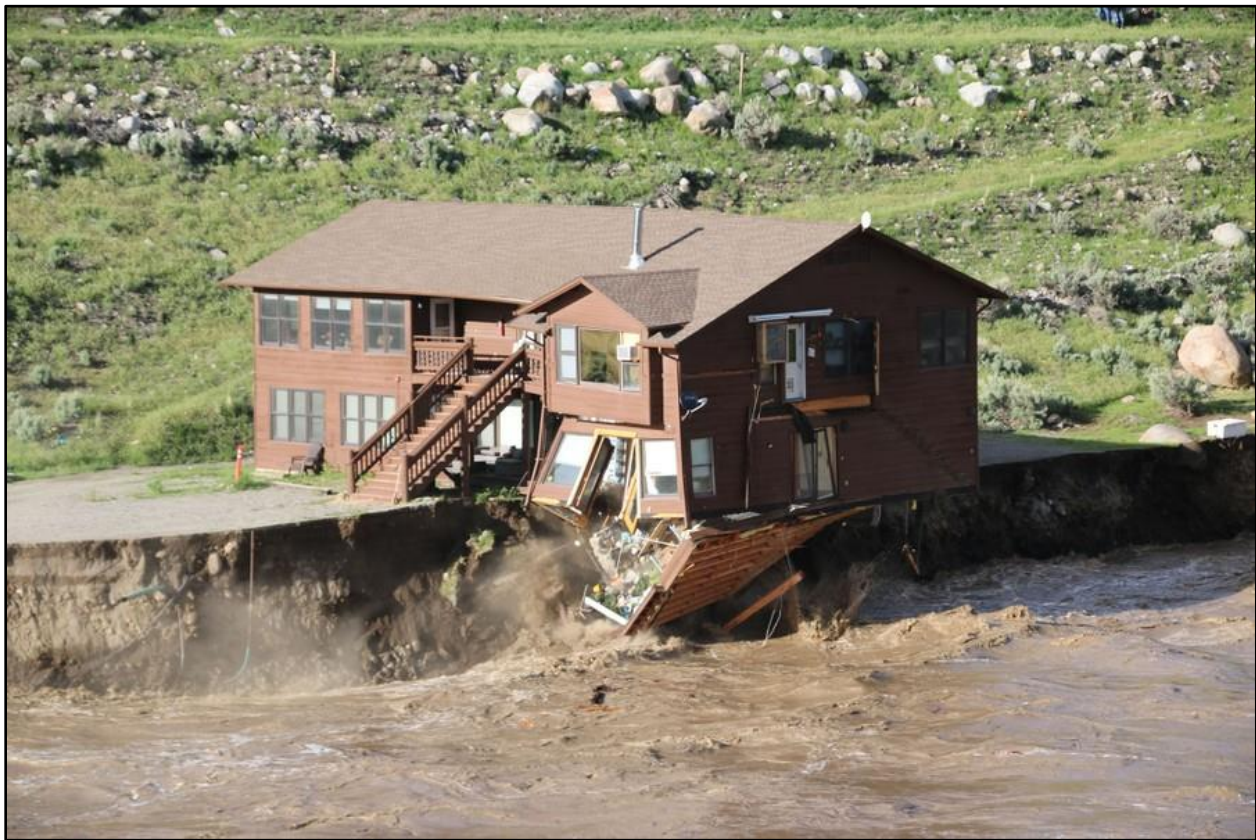
Figure 6. A National Park Service housing structure in Livingston, MT shown moments before falling into the Yellowstone River on June 13, 2022 (Gina Riquier / NPS).
