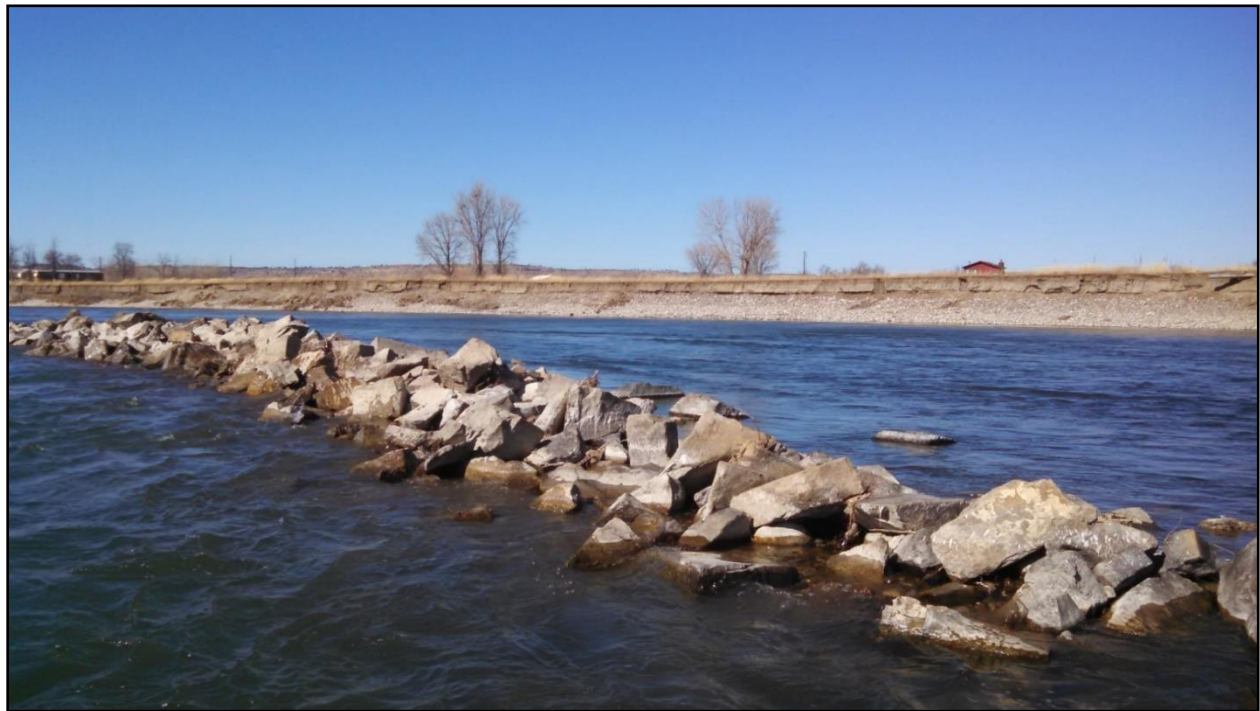
Figure 65. Failed bank armor (2011) in the middle of the Yellowstone River near Park City, MT where the bankline has rapidly eroded back towards the home in the background.
