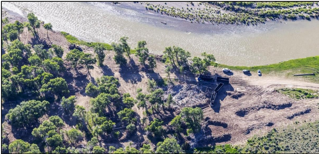
Figure 25. Woody debris removal from Yellowstone River floodplain following 2022 flood (Kestrel Aerial Services).
